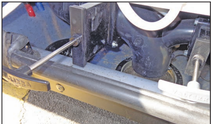
Figure 13-11: Sanitation coupling, valve and hose
