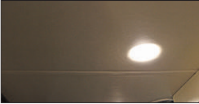
Figure 12-3: Typical ceiling in the Allegro Breeze
