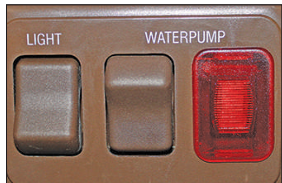
Figure 13-5: Water pump switch
