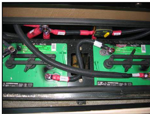
Figure 7-4. House Batteries (Underneath Entrance Door Step Well)
