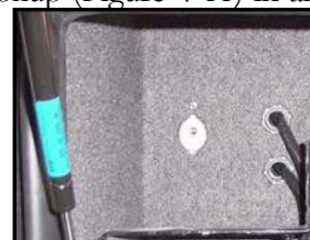
Figure 4-11. Cable & Telephone Jack
