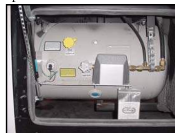
Figure 2-4. Liquid Propane Tank
