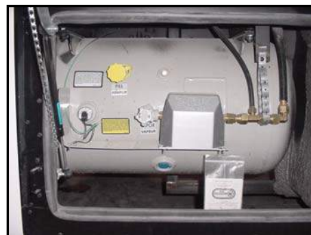
Figure 2-2. Liquid Propane Tank
