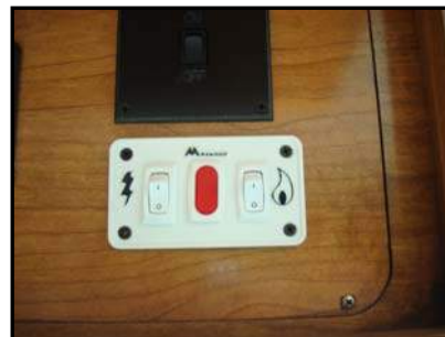
Figure 4-12. Water Heater Switches
