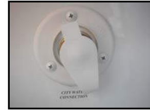
Figure 11-6. City Water Inlet
