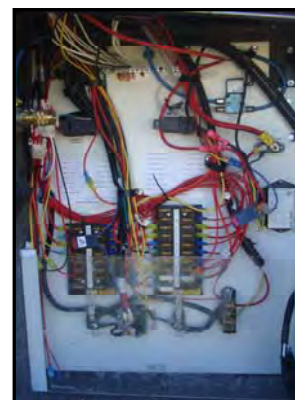
Figure 7-12. Fuse Blocks in exterior compartment on driver's side
