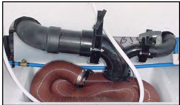
Figure 11-11. Sanitation Coupling, Valve, and Hose
