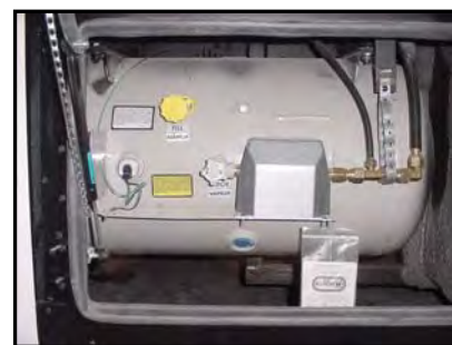
Figure 3-4. Liquid Propane Tank
