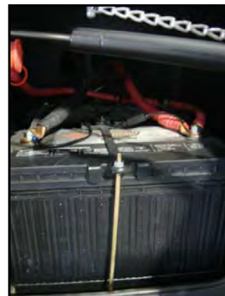
Figure 7-5. House Batteries (Underneath Entrance Door Step Well)
