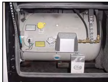
Figure 2-2. Liquid Propane Tank
