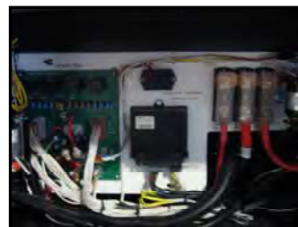
Figure 7-4. 12 VDC Battery System
