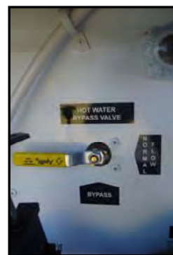
Figure 11-9. Water Heater Bypass System
