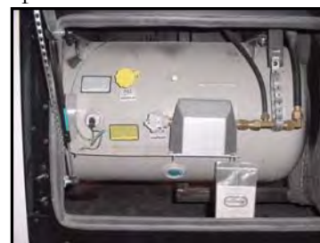
Figure 2-4. Liquid Propane Tank
