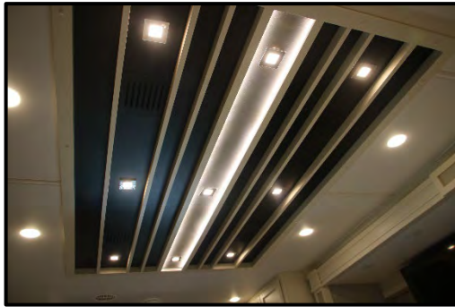
Figure 3-2: Outgoing/Return Air Vents
