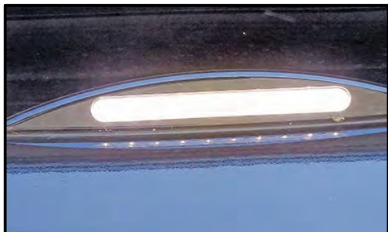
Figure 11-3: Exterior Security Light
