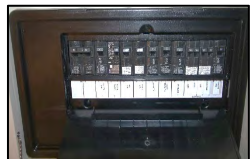
Figure 9-5: Circuit Breaker Box
