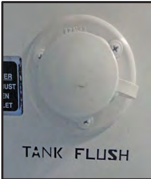
Figure 13-15: Tank Flush Connection
