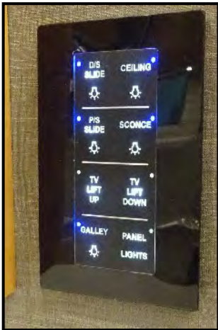
Figure 6-3: Television Lift Control Panel
