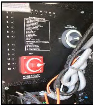
Figure 9-15 House Battery Panel
