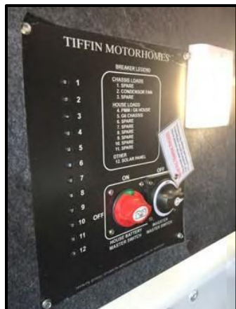
Figure 9-13: House Battery Disconnect Panel
