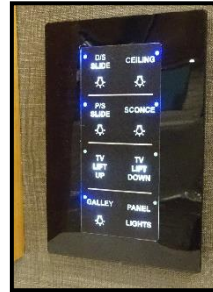
Figure 6-4: Television Lift Control Panel (located in the living room slide-out box)
