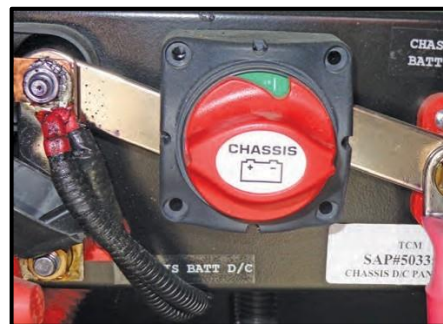
Figure 9-14: Engine Battery Disconnect Switch. Front Wall of Battery Camp
