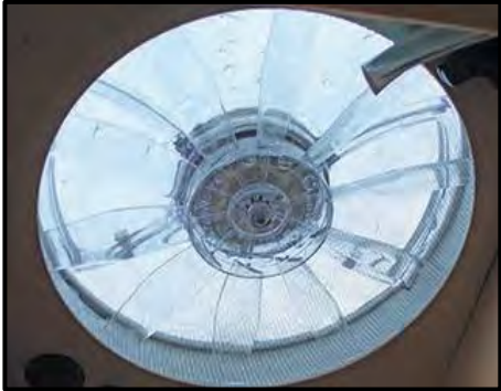
Figure 14-4: Overhead Vent Fan
