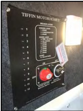
Figure 9-13: House Battery Disconnect Panel
