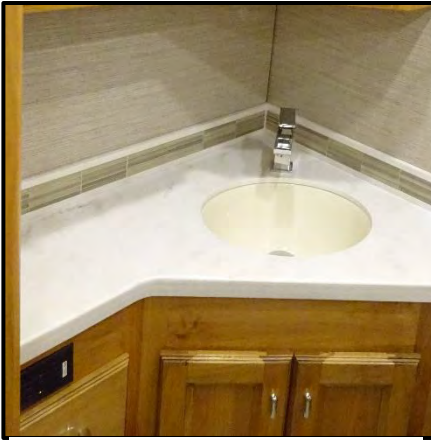
Figure 13-3: Bathroom Sink and Faucet
