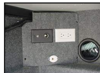
Figure 4-16. Cable & Telephone Jack
