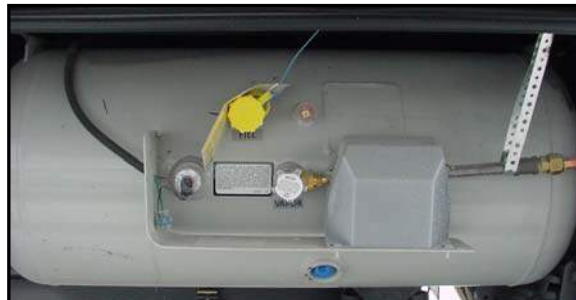
Figure 2-4. Liquid Propane Tank
