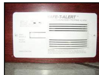
Figure 3-5. CO/LP Gas Detector
