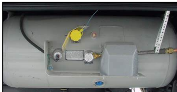
Figure 2-4. Liquid Propane Tank
