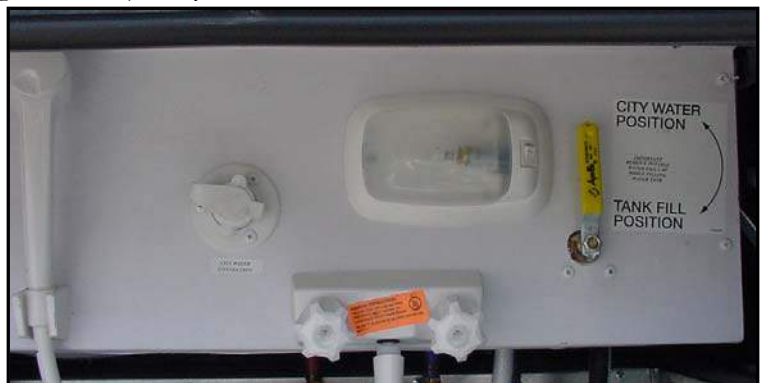
Figure 11-10. Exterior Shower in Sanitation Compartment
