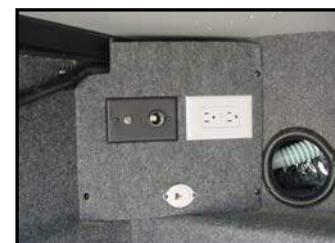
Figure 4-17. Cable & Telephone Jack
