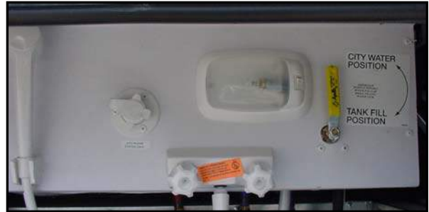
Figure 11-5. City Water Connection
