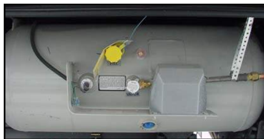
Figure 2-3. Liquid Propane Tank
