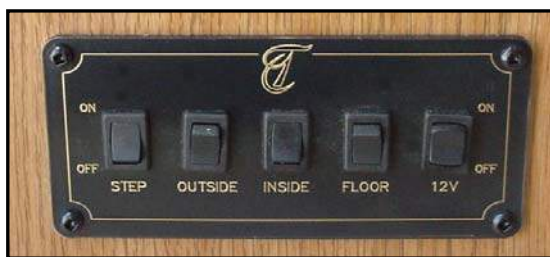
Figure 7-4. Battery Disconnect Panel
