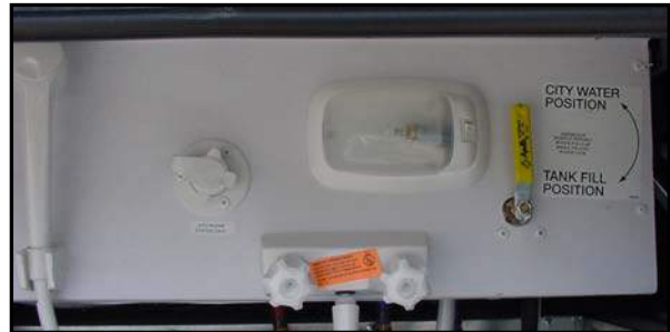
Figure 11-5. City Water Connection
