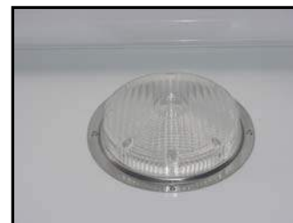
Figure 9-3. Security Light on Exterior
