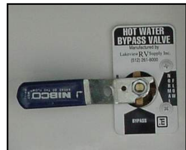
Figure 11-7. Water Heater Bypass Valve
