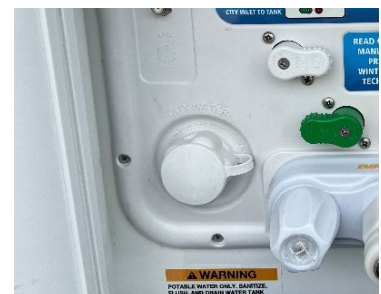
Figure 14-3: City Water Connection
