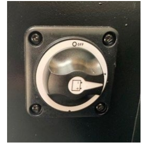
Figure 9-2: Battery Disconnect Switch
