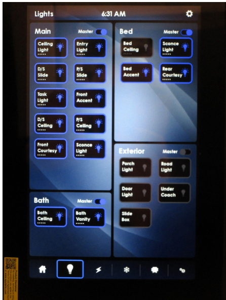
Fig. 12- 3 Spyder Light Controls in the Hallway
