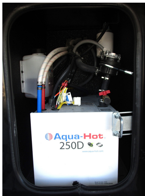
Fig. 3-4: Aqua Hot Heating System
