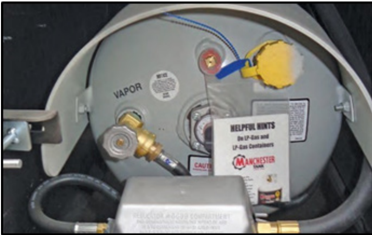
Fig. 4-1: LP Gas Tank
