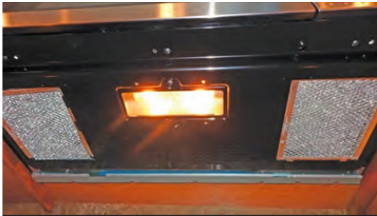
Fig. 5-5: Air Filtration Fan and Cooktop
