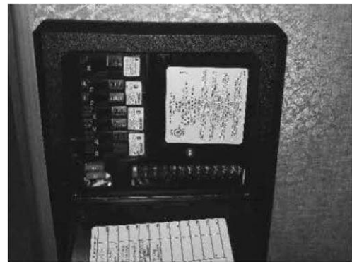
Figure 9-9: Main 120 VAC Load Center
