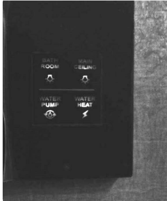
Figure 5-5: Water Heater Switch
