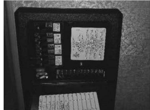
Figure 9-1: Circuit Breaker Box
