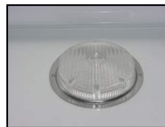
Figure 9-3. Security Light on Exterior
