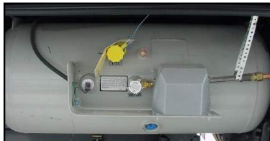
Figure 2-3. Liquid Propane Tank
