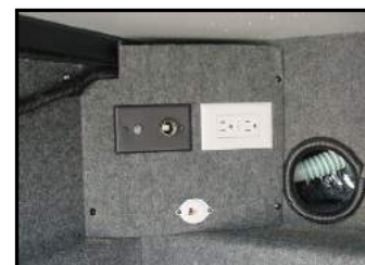
Figure 4-14. Cable & Telephone Jack
