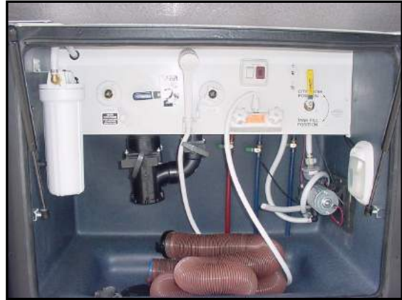
Figure 11-9. Sanitation Compartment with Wastewater Disposal Connection (Black Valve) and Wastewater Hose (Brown Hose)
