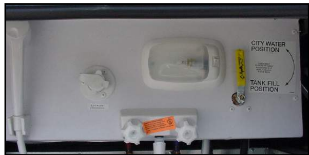
Figure 11-5. City Water Connection
