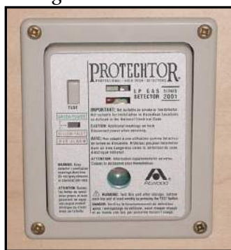
Figure 3-4. Propane Gas Detector
