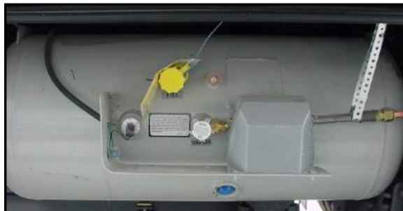
Figure 2-4. Liquid Propane Tank
