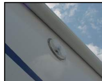
Figure 9-3. Security Light on Exterior
