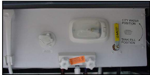
Figure 11-5. City Water Connection
