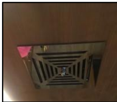
Figure 4-5: Return Air Vent
