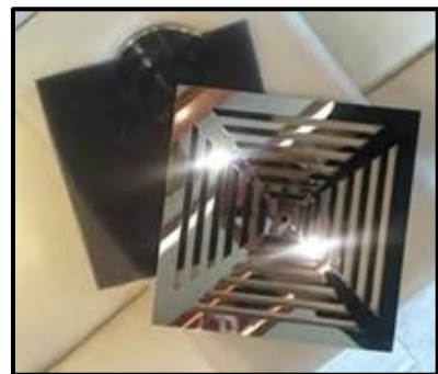
Figure 4-6: Air Vent Filter
