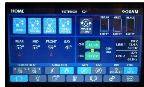
Figure 14-6: Spider Controls System Switch
