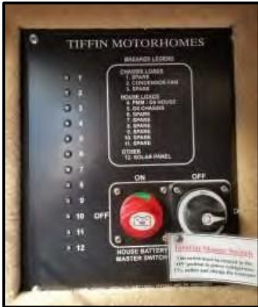
Figure 10-4: House Battery Disconnect Panel
