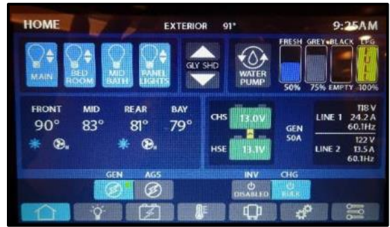
Figure 3-1: Home Screen for the Spyder Controls System
