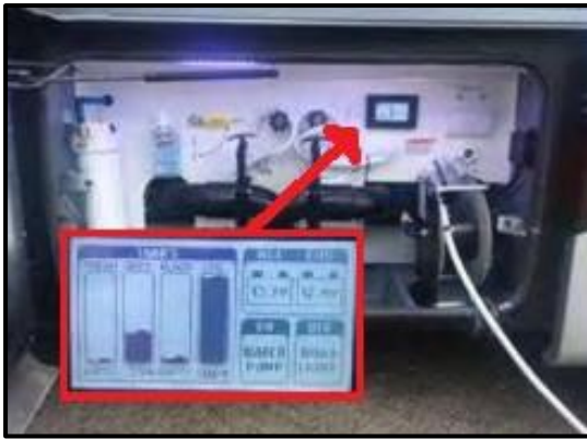
Figure 14-2: Location of Tank-Level Monitor in Plumbing Panel
