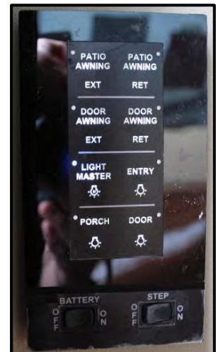
Figure 9-16: 12 VDC Disconnect Switch
