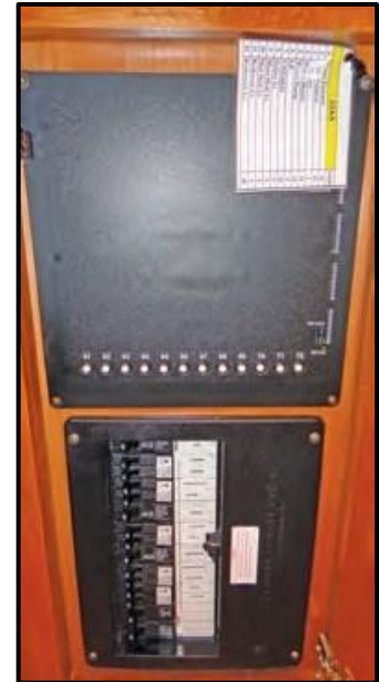
Figure 9-3: Circuit Breaker Boxes
