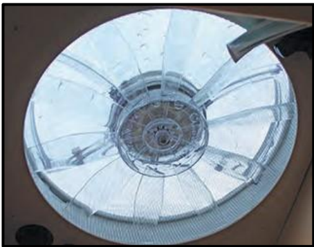
Figure 14-4: Overhead Vent Fan
