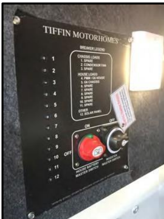
Figure 9-14: House Battery Disconnect Panel
