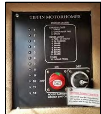
Figure 9-4: House Battery Disconnect Panel Switch
