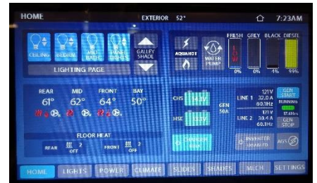
Figure 3-2: Home Screen for the Spyder Controls System
