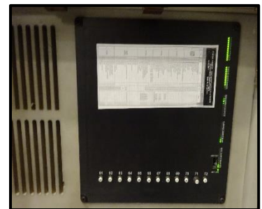
Figure 9-1: Circuit Breaker Box
