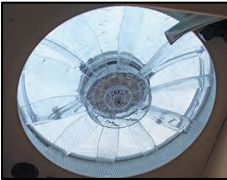
Figure 14-5: Overhead Vent Fan
