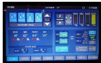
Figure 13-6: Spider Controls System Switch
