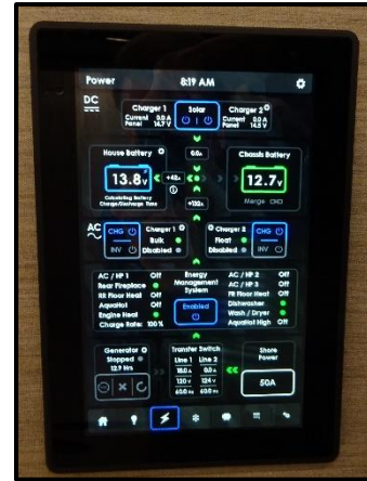
Figure 8-13: Control Panel for the Inverter/Charger
