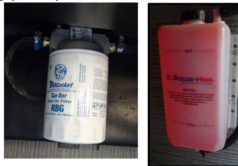
Figure 12-16: Aqua-Hot Surge Tank
