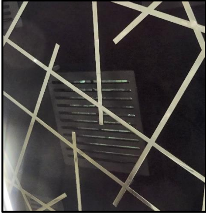
Figure 13-6: Overhead Vent Fan
