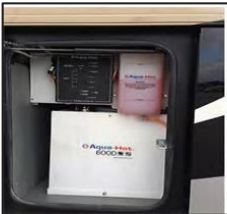
Figure 3-2: Aqua-Hot Surge Tank
