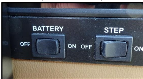
Figure 8-7: 12 VDC Disconnect Switch
