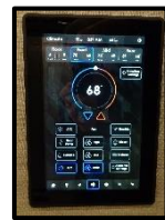
Figure 3-6: Heat Pump Controls
