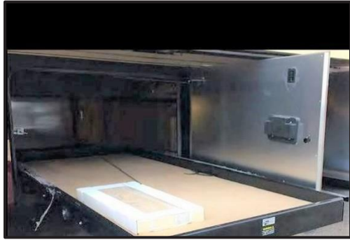
Figure 8-5: House Battery Disconnect Switch Location on the back of the DCD board
