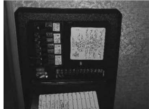
Figure 9-1: Circuit Breaker Box
