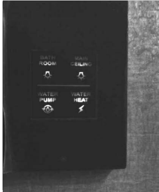
Figure 5-5: Water Heater Switch
