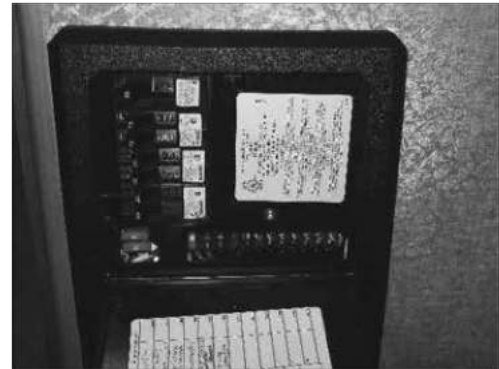
Figure 9-9: Main 120 VAC Load Center
