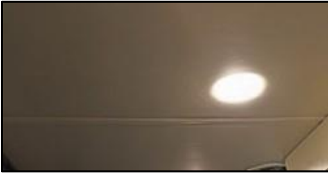
Figure 12-3: Typical Ceiling in the Allegro
