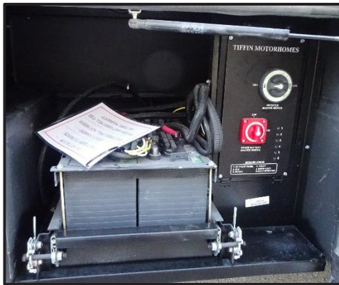
Figure 9-12: House Battery Disconnect Switch
