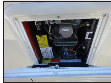
Figure 12-8: Water Heater Bypass System
