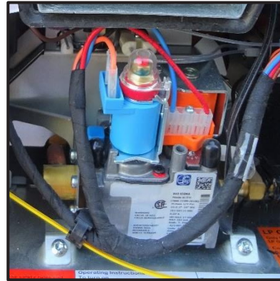
Figure 5-7: Water Heater Relief Valve
