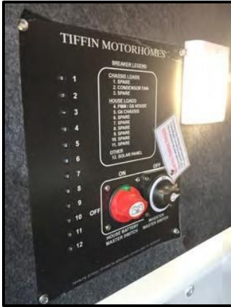
Figure 9-13: House Battery Disconnect Panel
