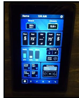
Figure 6-4: Television Lift Control Panel (located in the living room slide-out box)
