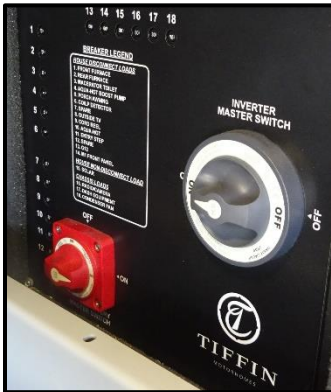
Figure 9-14: House Battery Disconnect Panel
