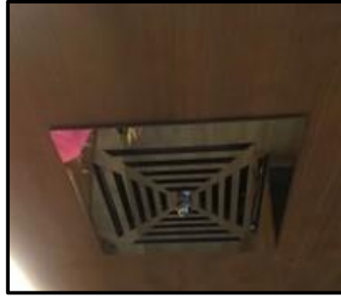
Figure 3-3: Return Air Vent
