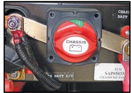
Figure 9-15: Engine Battery Disconnect Switch
