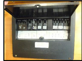
Figure 9-3: Circuit Breaker Boxes
