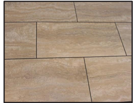
Figure 12-2: Typical Flooring in the Allegro RED
