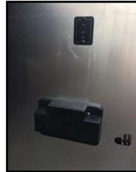
Figure 11-3: Electric Slide Tray Switch on Cargo Door
