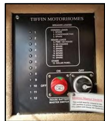
Figure 9-4: House Battery Disconnect Panel Switch
