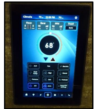
Figure 4-7: Heat Pump Controls
