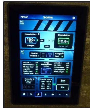
Figure 9-12: Energy Management System
