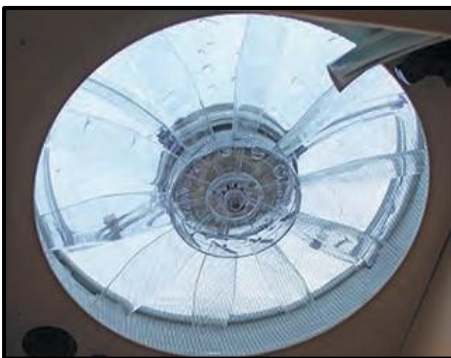
Figure 14-5: Overhead Vent Fan
