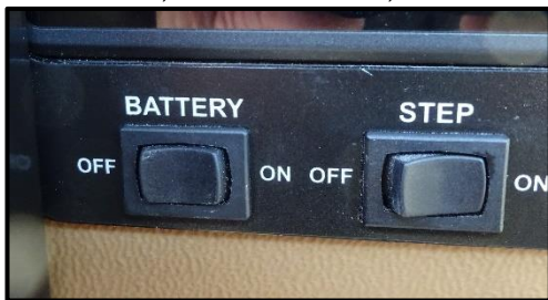
Figure 9-6: 12 VDC Disconnect Switch
