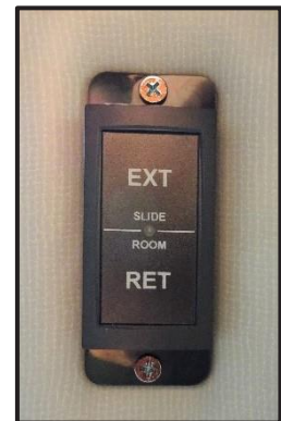
Figure 10-1: Front Slide-Out Switch
