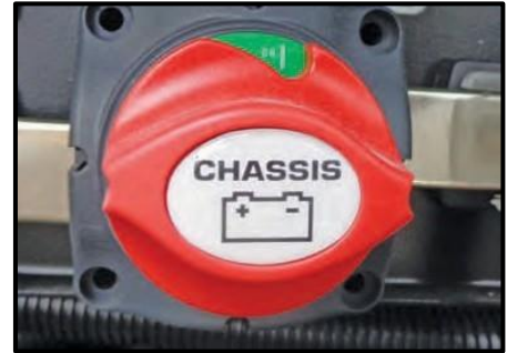
Figure 9-5: Engine Battery Disconnect Panel Switch
