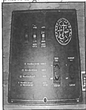
Figure 11-1. Monitor Panel (Water, LP Gas, Battery)
