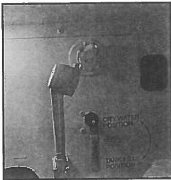
Figure 11-8. City Water Connection
