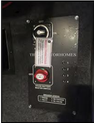
Figure 9-11: House Battery Disconnect Panel
