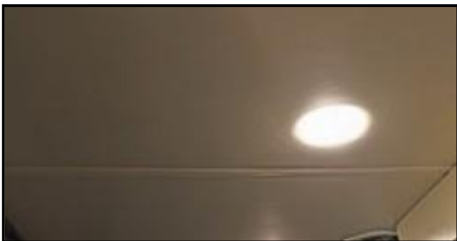
Figure 12-3: Typical Ceiling in the Allegro Breeze
