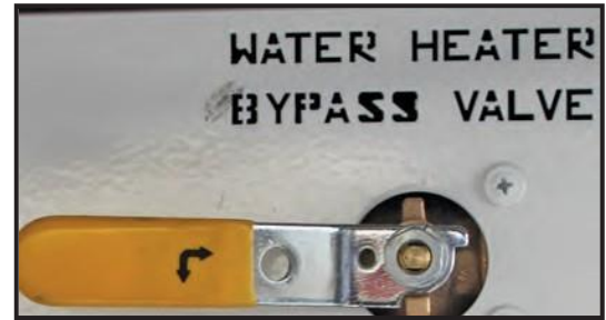
Figure 13-9: Water Heater Bypass System
