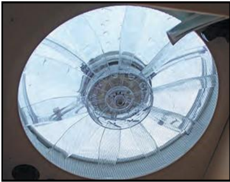
Figure 14-5: Overhead Vent Fan
