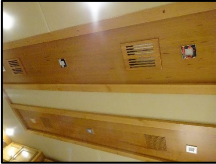
Figure 3-2: Outgoing/Return Air Vent
