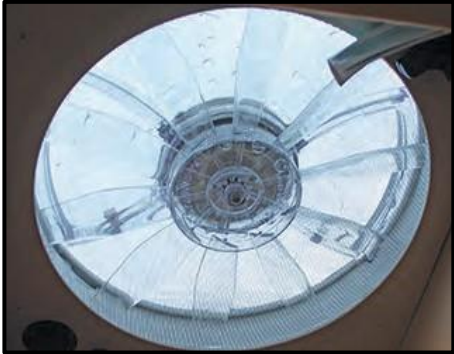
Figure 14-4: Overhead Vent Fan
