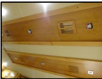
Figure 12-3: Typical Ceiling in the Allegro Bay
