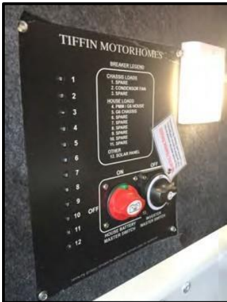
Figure 9-13: House Battery Disconnect Panel
