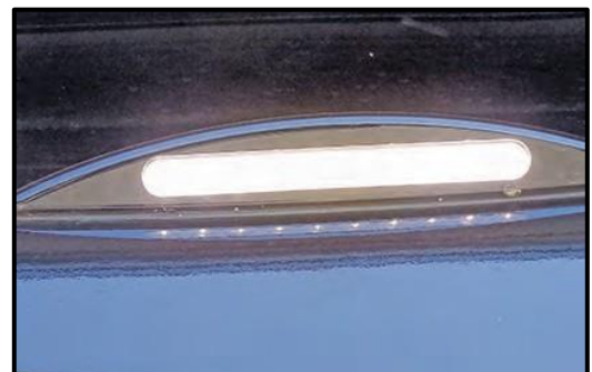
Figure 11-3: Exterior Security Light
