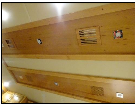
Figure 3-2: Outgoing/Return Air Vent
