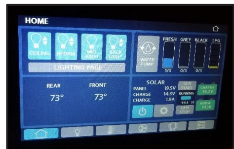
Figure 13-5: Spider Controls System Switch
